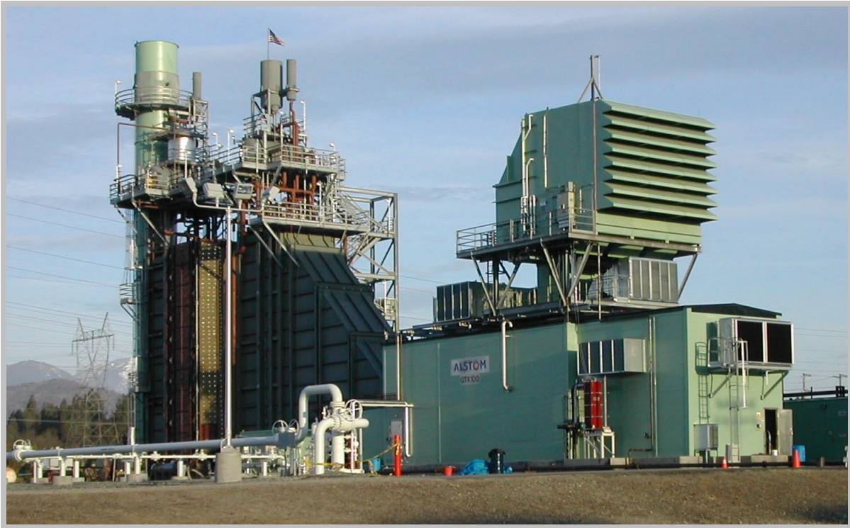
Redding's Generating Unit No. 5: The Pioneer Combined Cycle installation in the U.S. of the Alstom GTX100 combustion turbine
